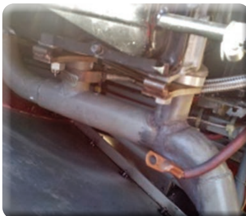
Loose ground strap very visible after removing cowl. Bolt completely gone.
